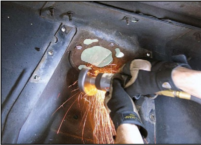
With the upper spring seat removed, a grinder is used to smooth flush any remnants of the original spot welds.
